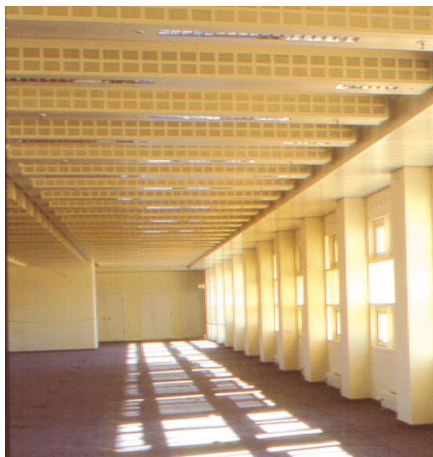
Figure 6: Mixed mode building showing chilled beams.
