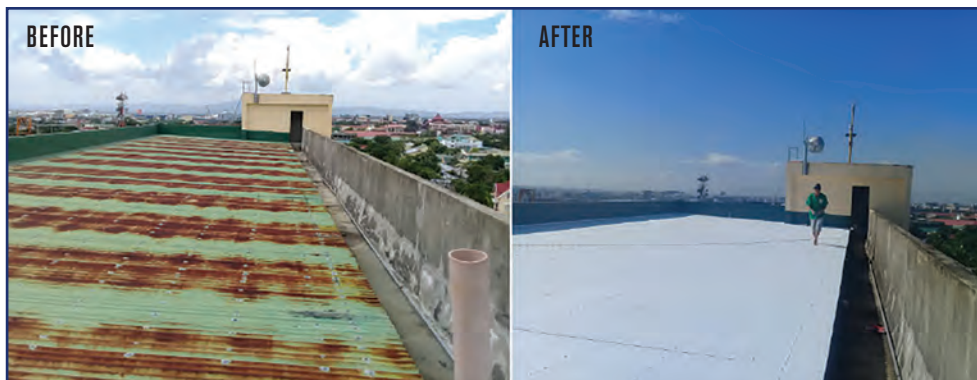
The roof at Naga College in the Philippines before (left) and after (right) becoming a cool roof, which reduces the absorption of external heat and the need for air conditioning in buildings.
