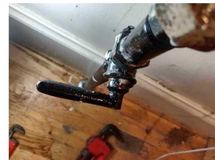
Fig 6. A leaky shutoff valve observed in the field
