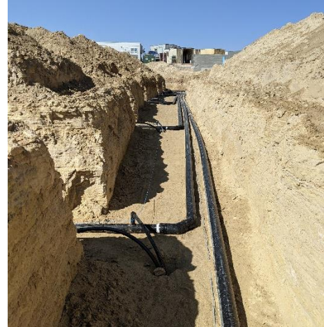
FIGURE 7: Ground Heat Exchanger
