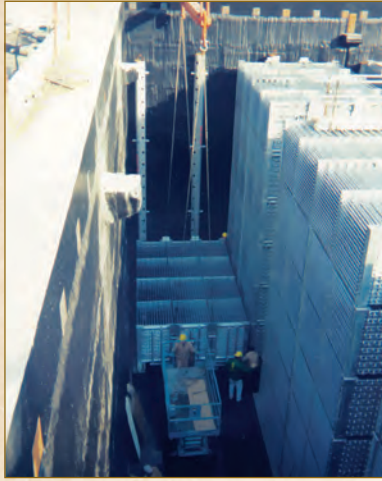
PHOTO 7 Northwind Chicago Plant #2 under construction with external melt ice-on-Coil units. (courtesy Enwind Chicago)
