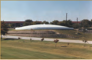
PHOTO 3 Texas Instruments CHW TES. (courtesy DN Tanks)
