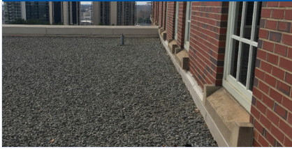
FIGURE 5 A roof setback halfway up the building can provide space for supplemental mechanical equipment.
