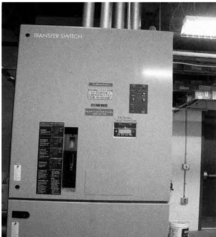
Figure 10-3 Emergency Load Transfer Switch
