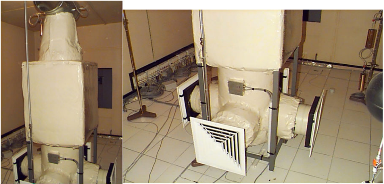
Figure 13-24 Heating and air-distribution system (left); diffusers close-up (right).
